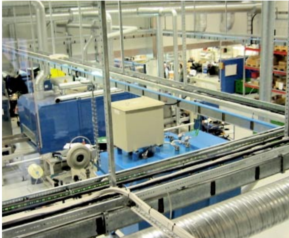
The new brazing facility in Västerås, Sweden is a center for CuproBrazed research and development activities.
